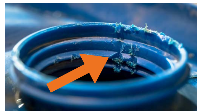
Flange cracked, threads stripped, or weld is broken
